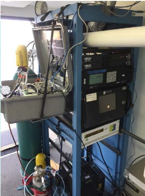
'Laboratory Grade System' Instrumentation In Trailer
